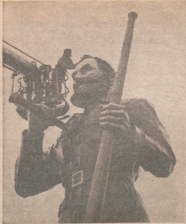
COMMUNITY RELATIONS —The face of Bangor's Paul Bunyan receives a touch up by Mr. J. Norman Martin of Tom Kane Advertising. The job was recently completed when city officials noticed that the paint had begun to chip and asked Dow to furnish a de-icer to use on the job. The OMS de-icer is operated here by TSgt. Robert E. Dickens.
